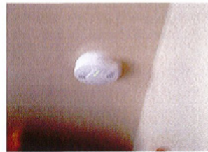
Smoke detectors are not interconnected with other smoke detectors in the building
