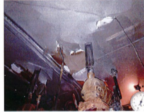
Moisture-damaged, collapsing ceilings in basements
