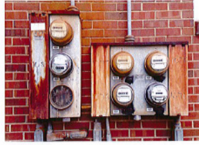
Corroded electrical equipment with water entering at service connection point
