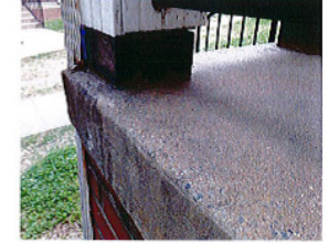
Rusted patio and porch rails
