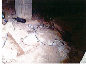
Evidence of moisture in crawlspace/basements
