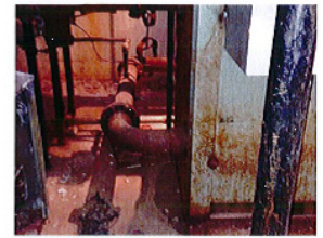
Severe corrosion of systems
