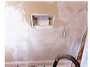
Washer connection tied to an undersized 3" galvanized water system which is inadequate
