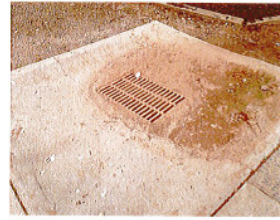
Erosion and blockage at drains
