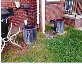
Outdated compressor units
