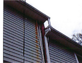
Vinyl siding is 20+ years old and in poor condition
