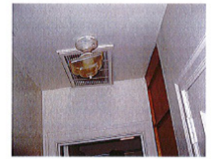
Non-working and/or unsecured fixtures
