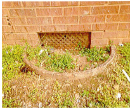
Erosion and blockage of drains
