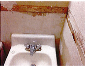
Water penetration in units
