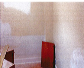
Lead-based paint is painted over and not abated
