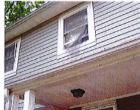
Unsecured and/or damaged windows
