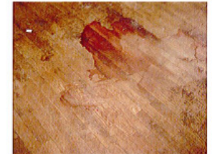
Evidence of moisture below the floor joists and water damage
