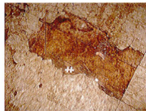
Moisture penetration in the floor joists creates dangerous situations in the units
