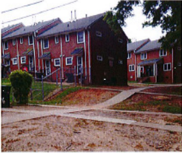
Severe erosion and sidewalks with hazardous cross-slopes
